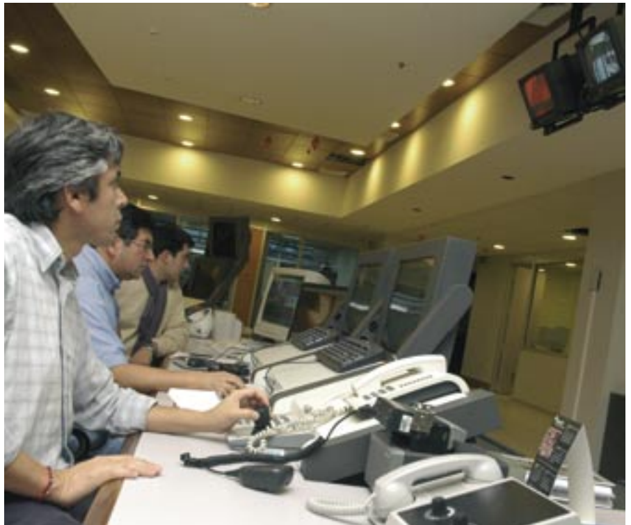
Control Room at the Santa Fe Mill
